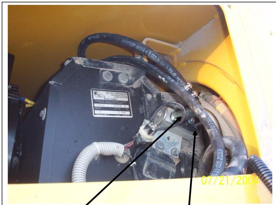
1/2" fitting attachment to expansion valve with "H" clamp
