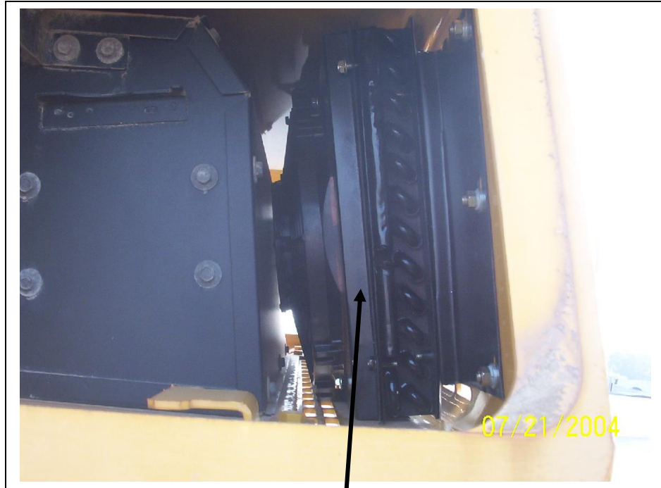
Condenser mounted to its screen frame and bolted back onto the cab.
