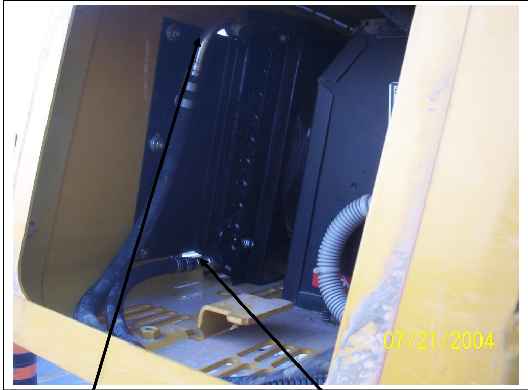
13/32" fitting on condenser
